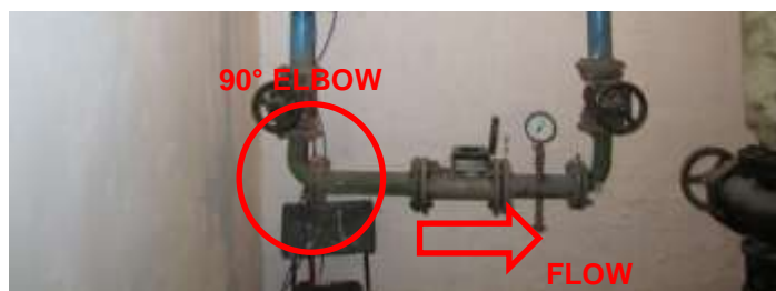
Figure 27 : Metering point configuration before the STV unit (NON-DOM #6)
