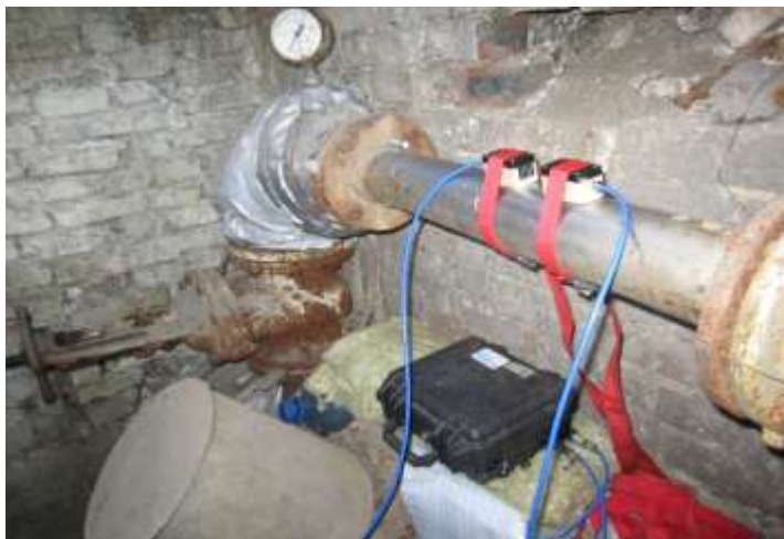
Figure 16 : Portable ultrasonic flowmeter installed in S.A. BUCURIA
