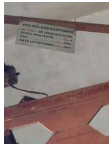
Graph 11: Expired crane inspection label
