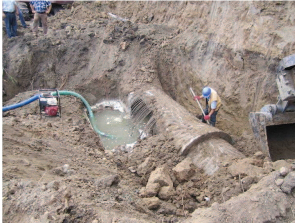
Figure 19: Burst on a ND1200 cement pipe threatening the road
