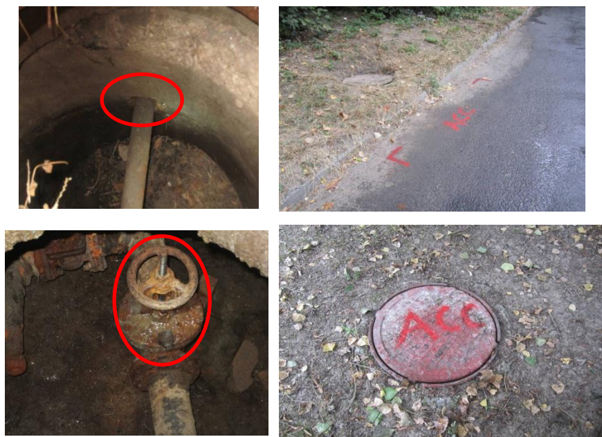
Figure 17 : Unrepaired leaks reported as solved by operational sectors
