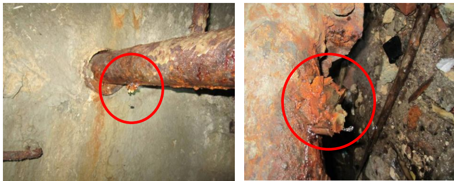
Figure 18 : Leaks still active after repair
