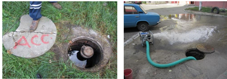
Figure 22 : Network manholes full of water
