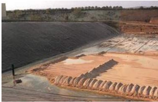
Figure 22 View of a landfill cell during the construction phase; note the drains and the geotextile.
