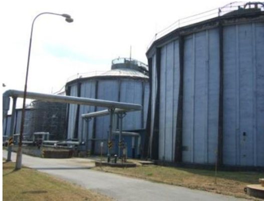
Figure 16 Digesters at Prague WWTP (Czech Republic)
