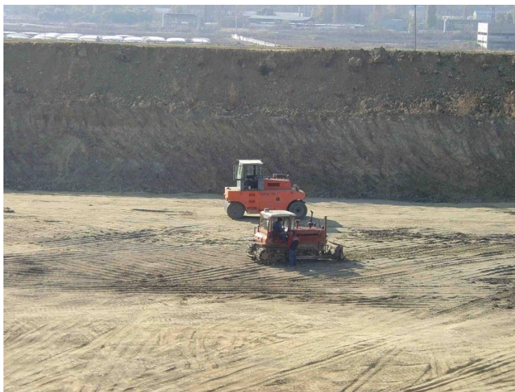
Figure 12 Construction of a sludge pit (November 2011) at Chisinau WWTP. Geotubes can be seen in the background.
