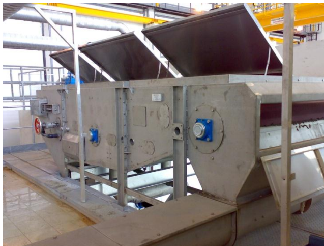
Figure 17 Gravity belt-thickener Flavy, implemented at the Pest-South and Pest-North WWTPs.
