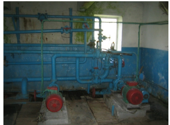
Pump downstream the reservoir
