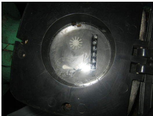
Flow meter downstream the pump
