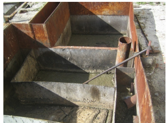
Grease trap after each production unit
