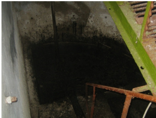
Collection pit for all wastewater streams before transfer to the sewerage system (where samples are taken by ACC).
