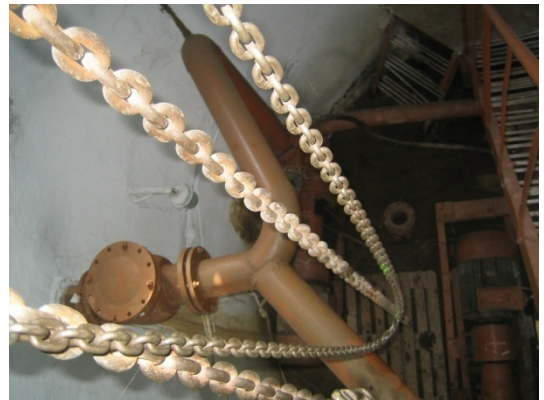
Pipe to the sewerage system downstream the transfer pump.
