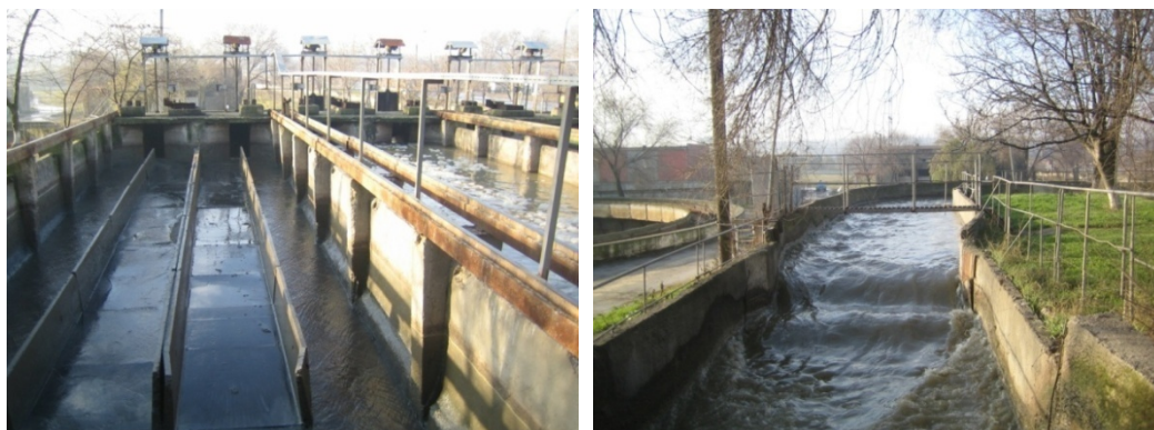
Figure 16: Photos: Sand removal tanks. The water normally flows from the front to the back. During backwashes the water flow backward and washes the sand away to a sand trap (in front of the tank; not shown in the picture). (left) & Open channel which connects the sand removal tanks to the splitting chamber located upstream the primary settlers. (right)
