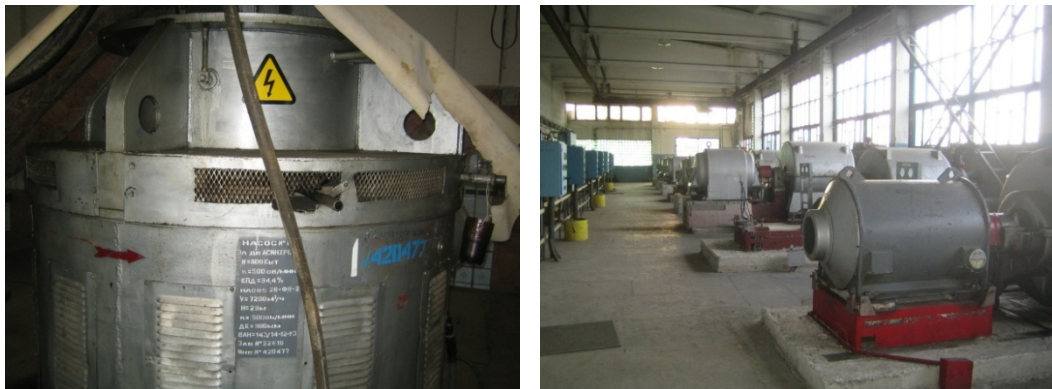
Figure 32: Photos: Lift pumps in the fine screen building (left) & Centrifugal blowers (right).
