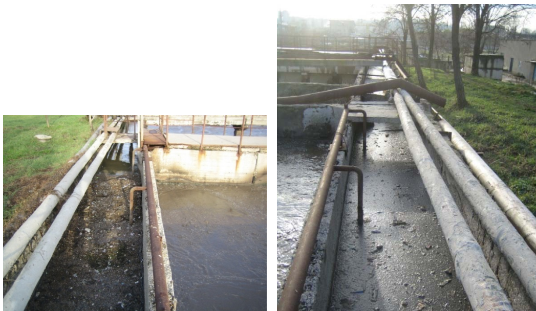
Figure 29: Photos: Stagnant sludge (left) & Wastewater in idle open channels (right).
