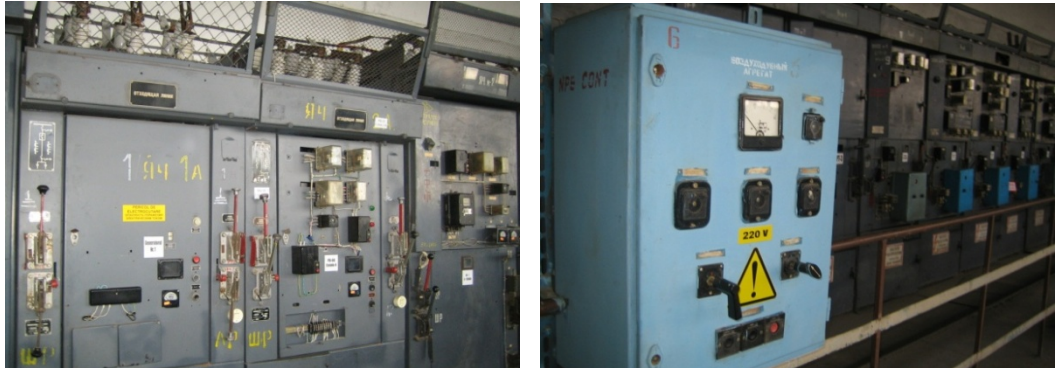
Figure 33: Photos: Examples of the electrical installation.
