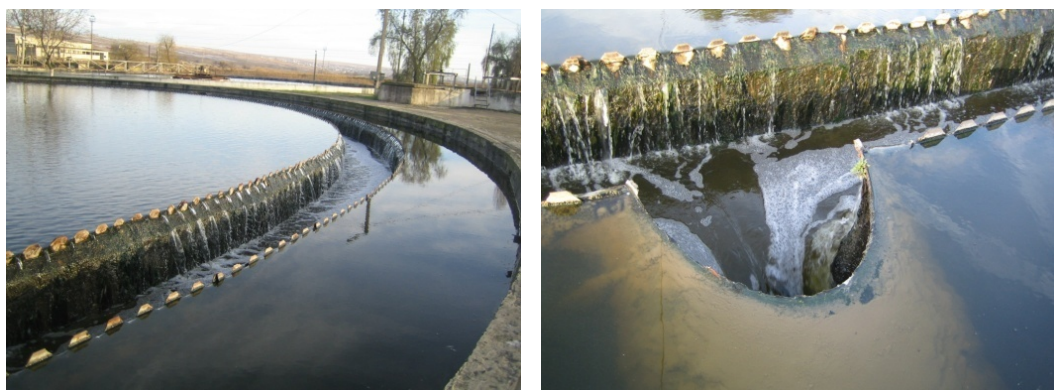
Figure 24: Photos: Channel of clarified water. (left) & Clarified water exit point. (right).
