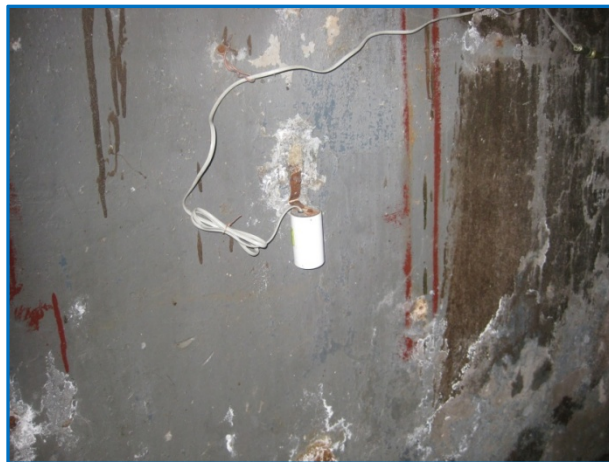
Figure 2: High Level Chlorine Gas Detectors
