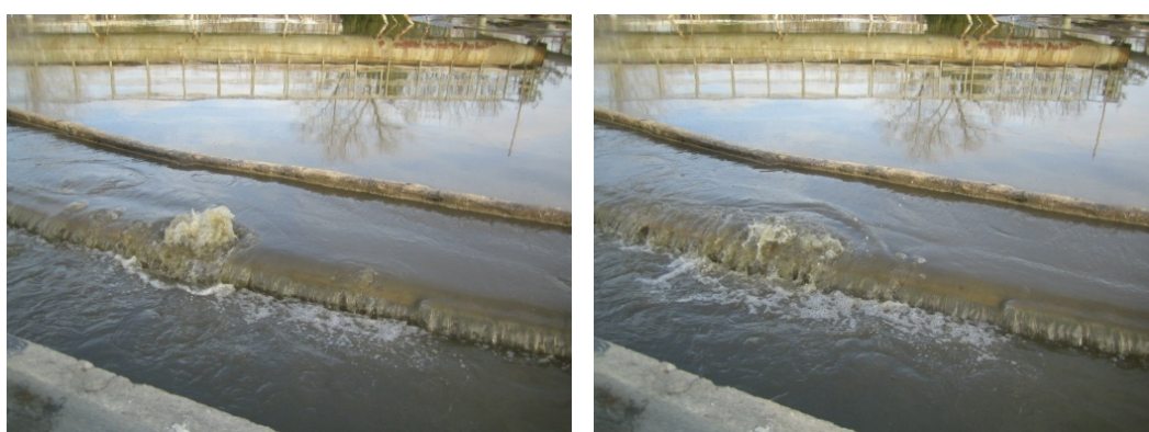
Figure 18: Photo: Hydraulic issue in one of the primary settling tank (inlet of the pretreated wastewater)
