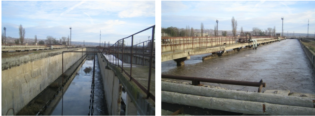
Figure 21: Photos: Decommissioned aeration channel. Note the aeration system at the bottom of the tank.(left) & Aeration channel (stabilization zone).
