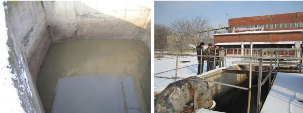
Figure 12: Photos: First inlet chambers, where the two sewers from the city meet (left) & Second inlet chamber (right)
