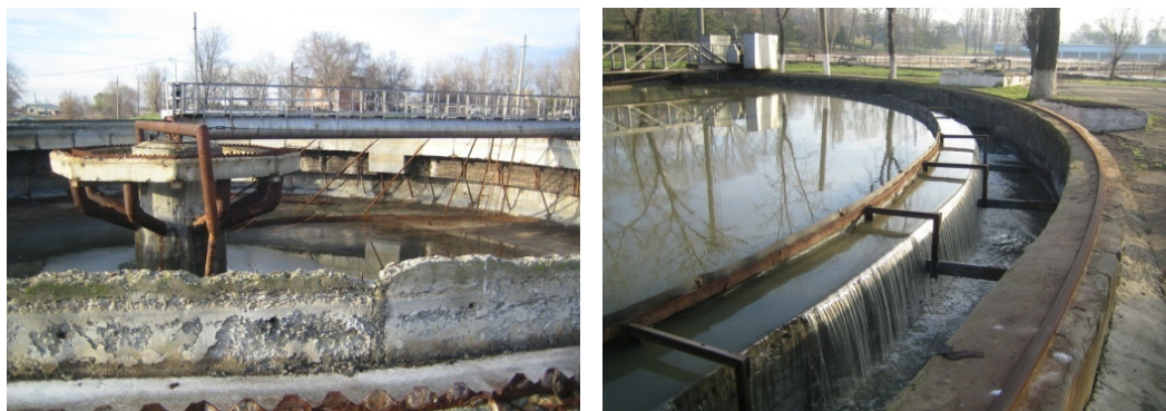
Figure 17: Photo: Decommissioned primary settling tank. (left) & Primary settling tank in operation. (right)
