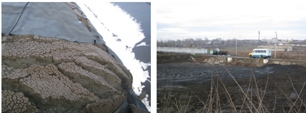
Figure 28: Photos: Opened Geotube prior to sludge handling. (left) & Sludge is taken out of the Geotubes and transported to a final disposal site nearby. (right).
