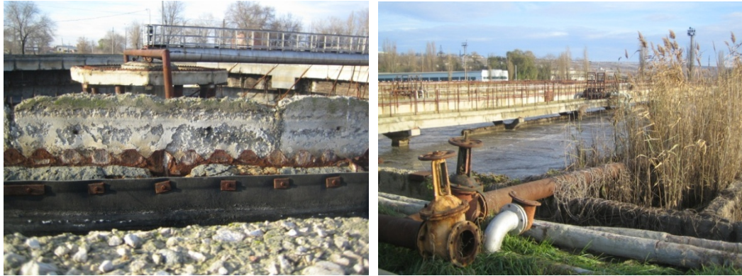
Figure 31: Photos: Degraded concrete structure in one primary settler (left) & Vegetation has grown in idle channels (right).
