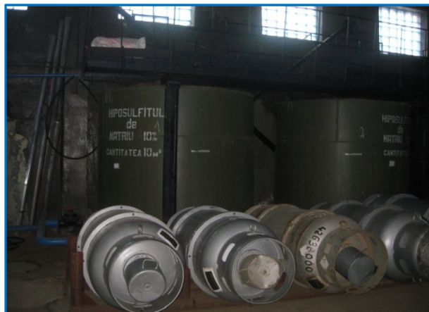
Figure 1: Chlorine Gas Drums with Long Gas Lines
