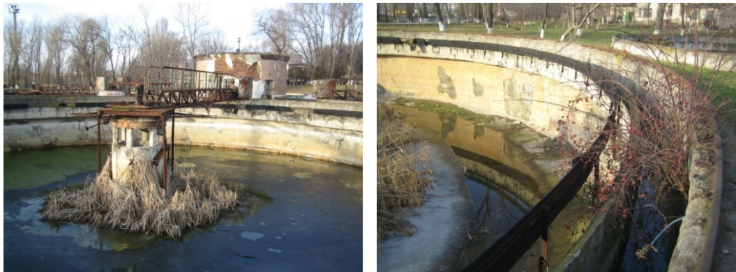
Figure 25: Photos: Static sludge thickener
